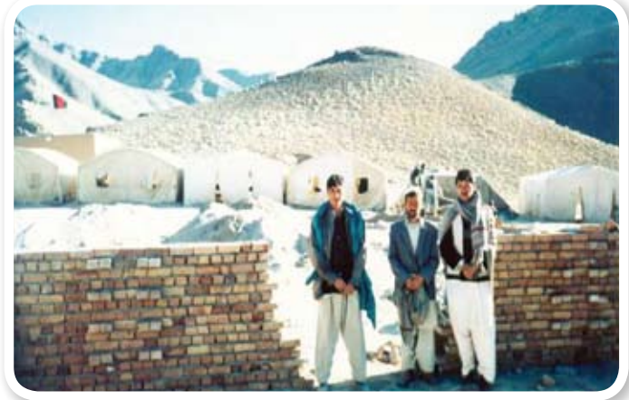
In the background are the tents where the children have been attending school for the last 8 years. This wall is part of the new school which is nearly complete. The children are so excited! The village provided the land for free.
